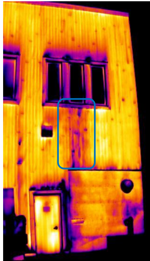
Figure 7. Moisture entering the wall system below a window, showing a cool pattern as the wall warms after sunrise.
